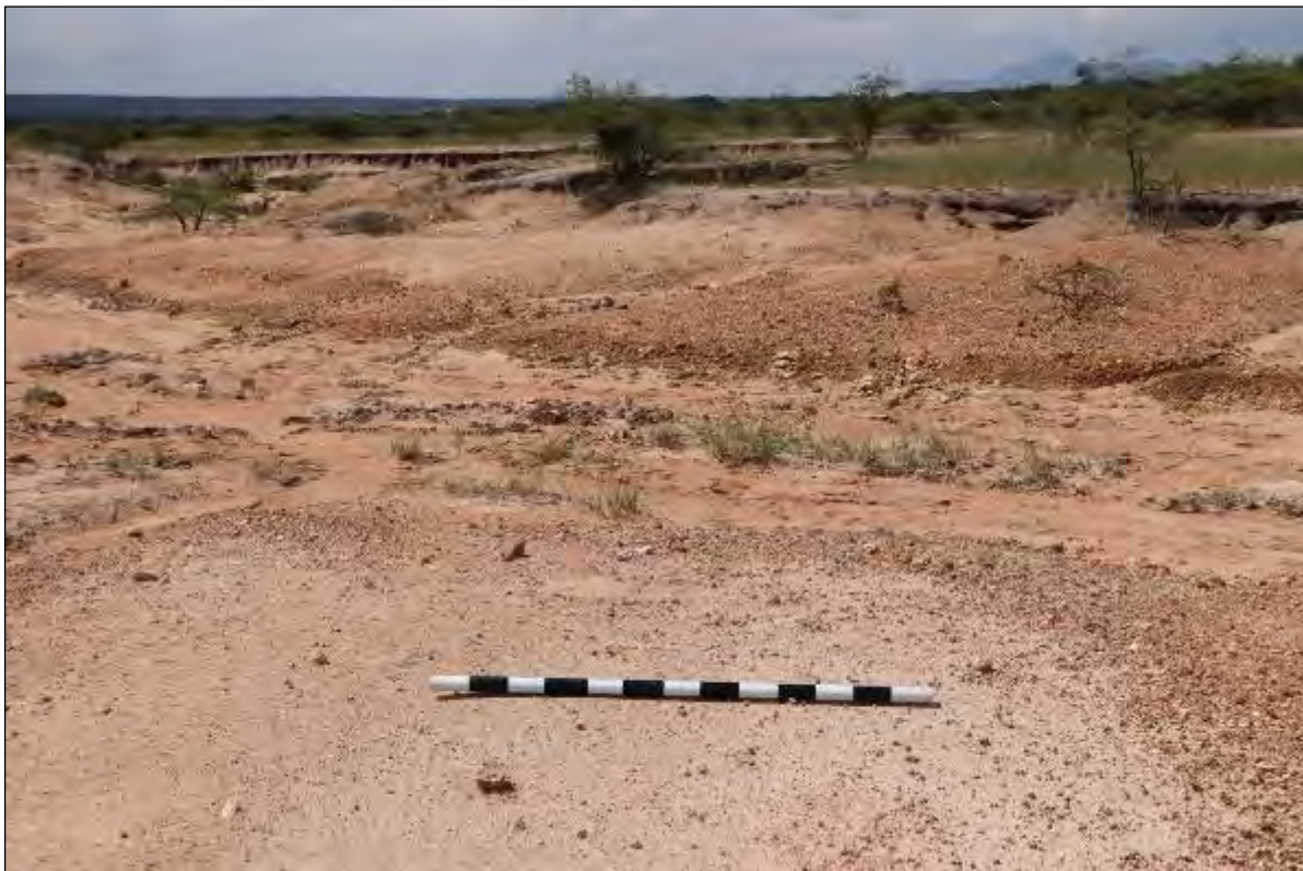
Figure 6 – Eroded watercourses such as the one depicted here are found in both the North WRD and Blinkwater TSF areas. The watercourse shown here is from the North WRD area.
