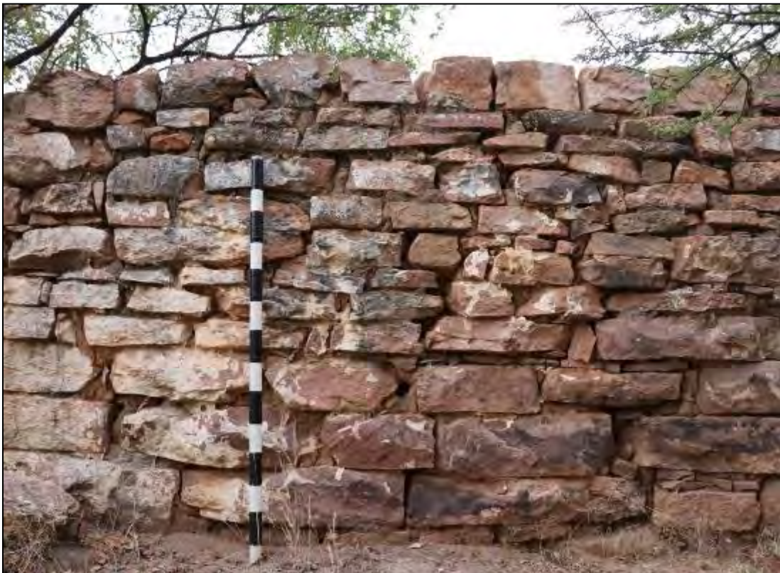
Figure 116 – Section of reasonably well-preserved walling on the western side of the farmhouse. Scale in 10cm increments.
