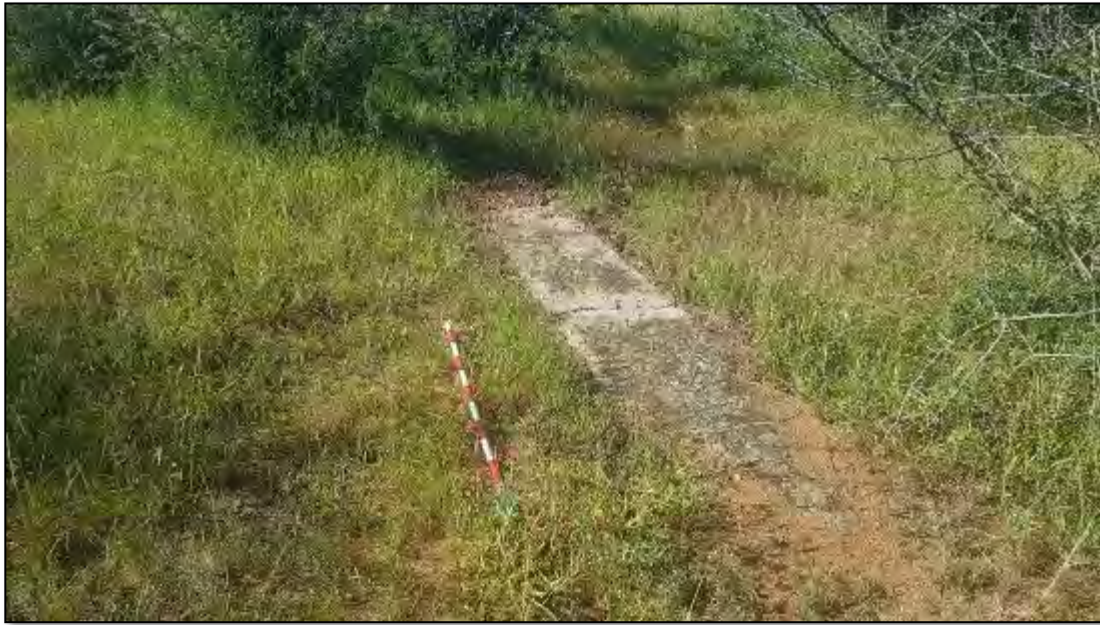
Figure 87 – General view of the site showing a section of the concrete foundations. Scale is in 10cm increments.
