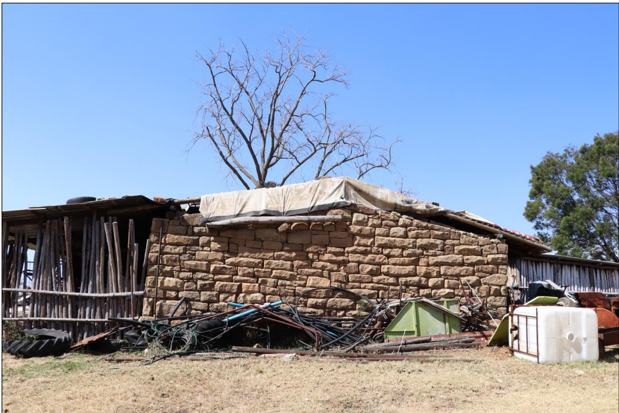
Figure 64 – General view of the second sandstone dwelling located at site KCP 18. The scale is in 10cm increments.
