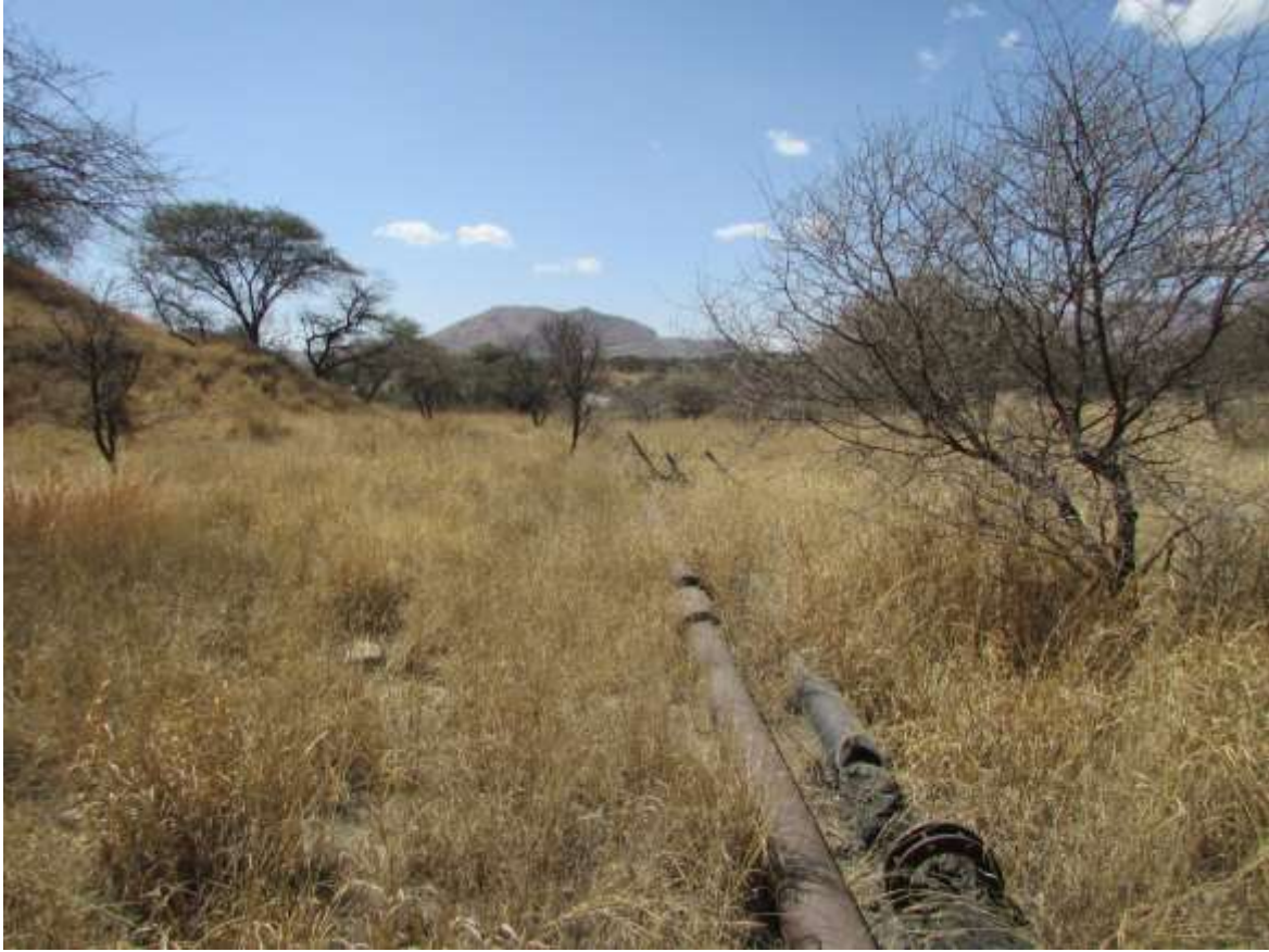
Figure 6: Old pipeline in the TWF3 area.
