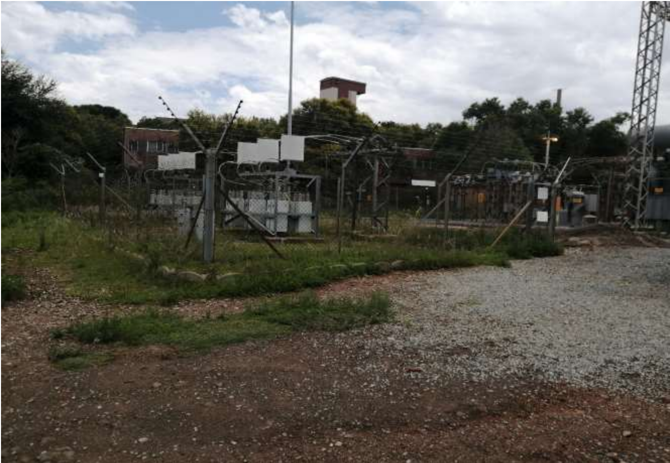
Plate 1: Showing the substation associated with the proposed development.
