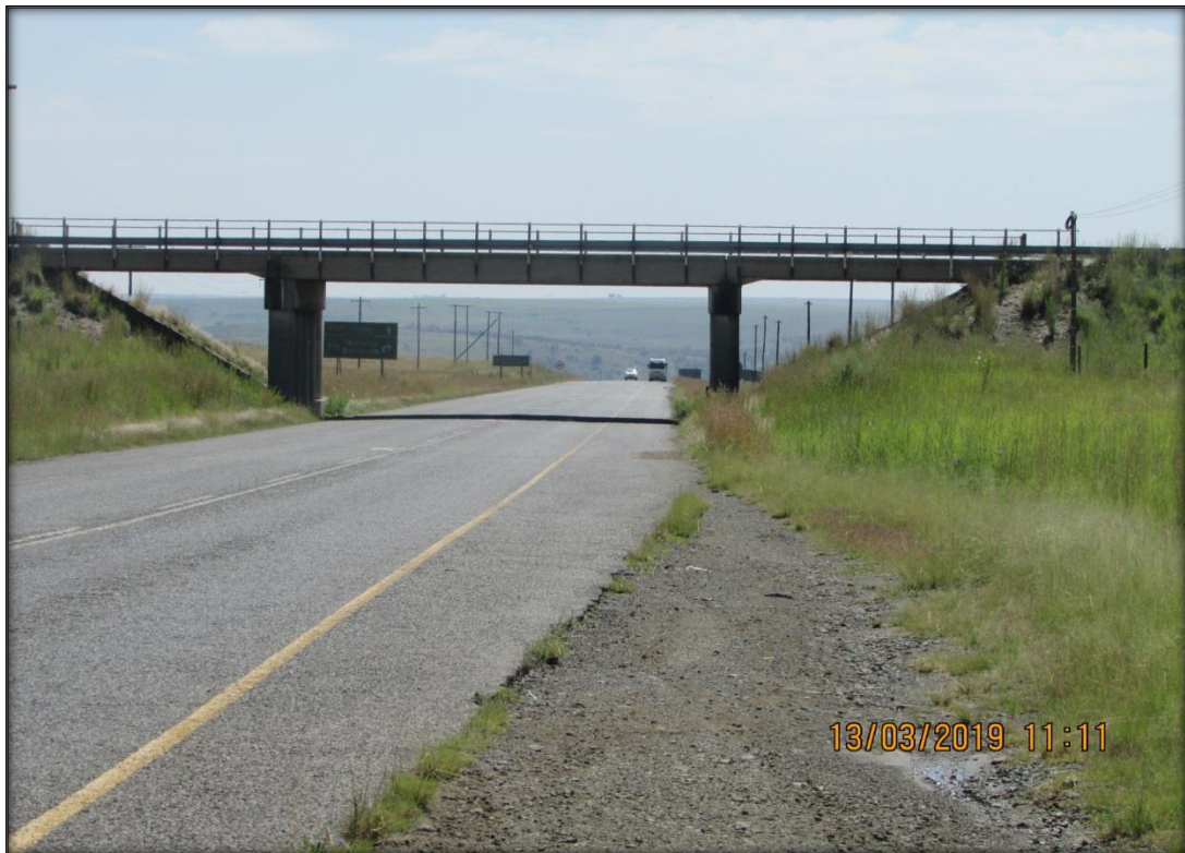
Figure 16: View of one of the bridges on the route. This bridge is fairly recent in age and of no heritage significance.
