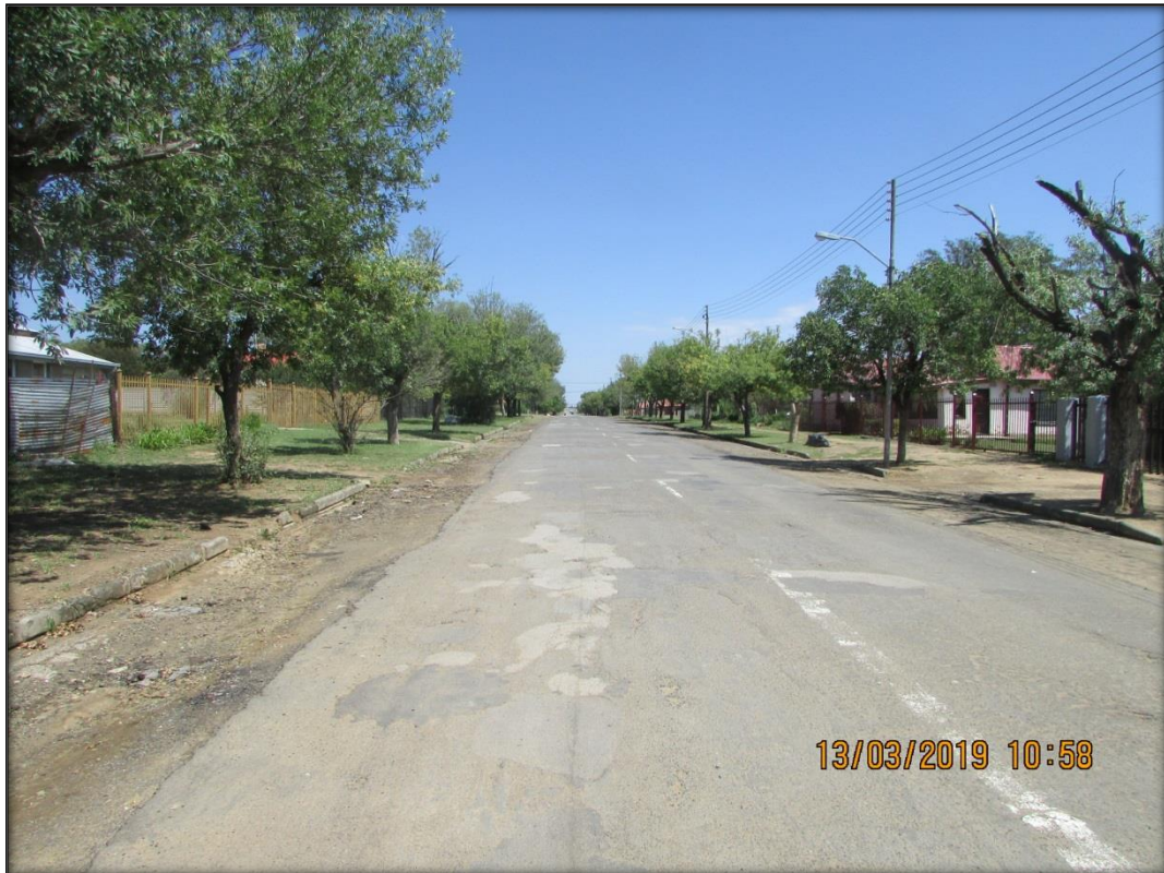
Figure 13: A section of the pipeline route follows an existing road through Lindley.
