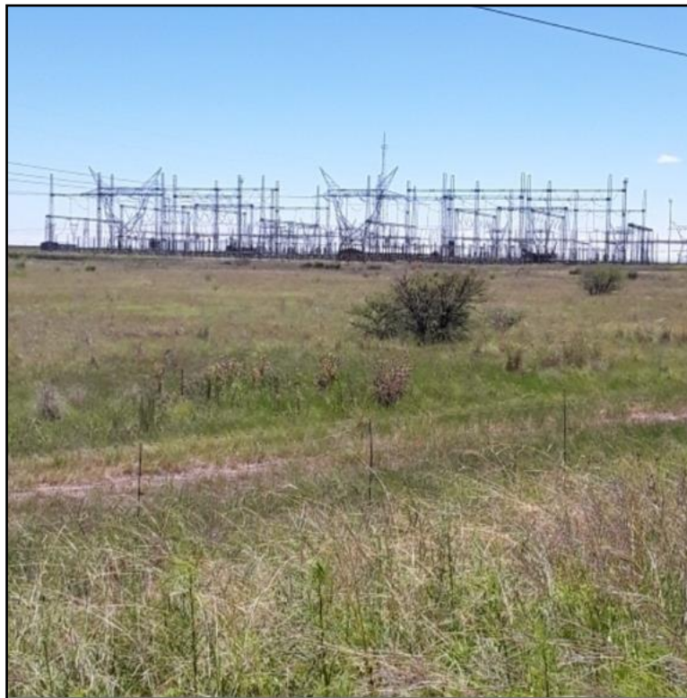
Figure 31:View of the existing Theseus substation northeast of the Doornrivier PV 1 Facility.
