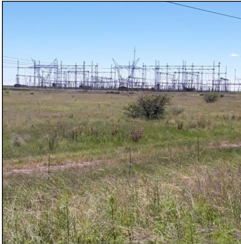
Figure 31:View of the existing Theseus substation northeast of the Doornrivier PV 1 Facility.
