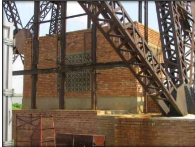
Fig.28: Close-up of Headgear and electrical substation. This feature will also be kept intact.
