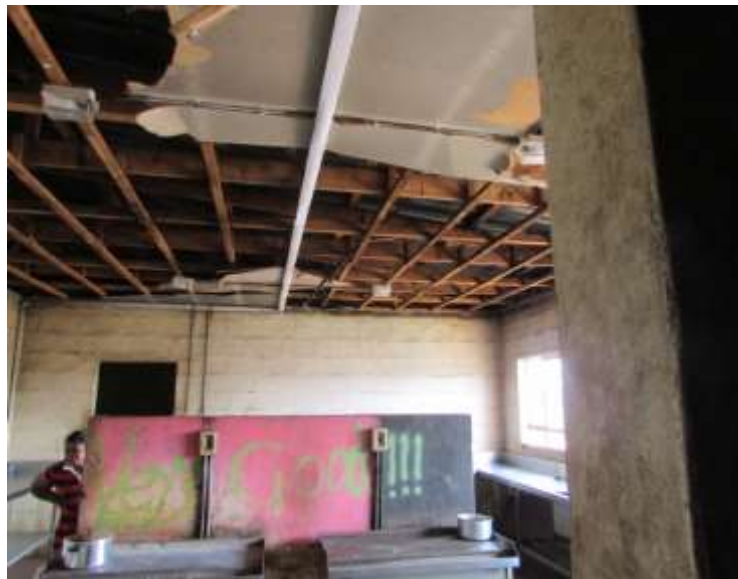
Figure 12: One of the communal kitchen areas. Note the roof damage. There are 8 such areas per Block (4 per floor).
