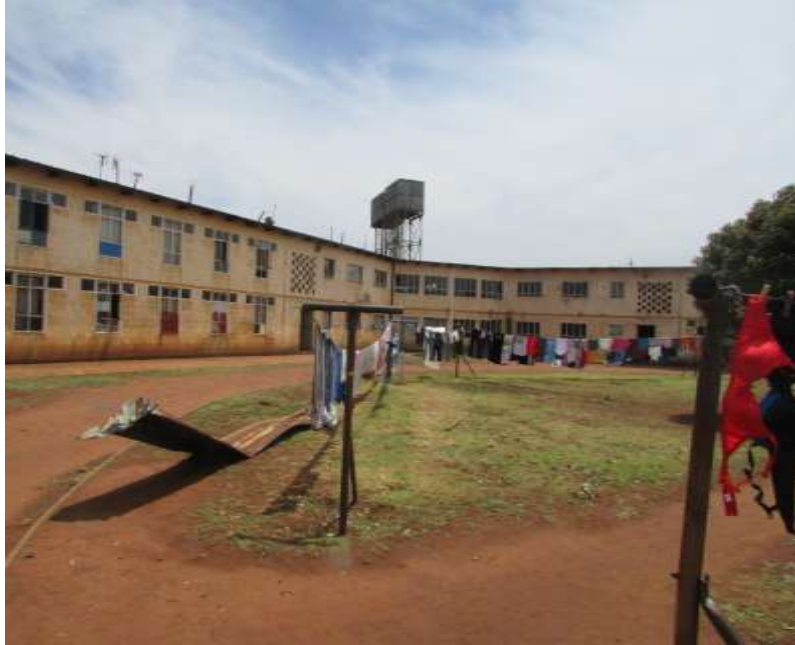
Figure 7: A view of the inner public space in Block C. Note the corrugated iron roofing blown off during a recent storm.
