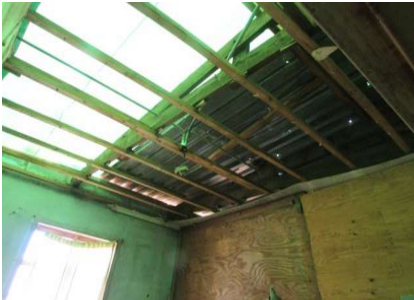
Figure 10: Roof damage caused by recent storms.
