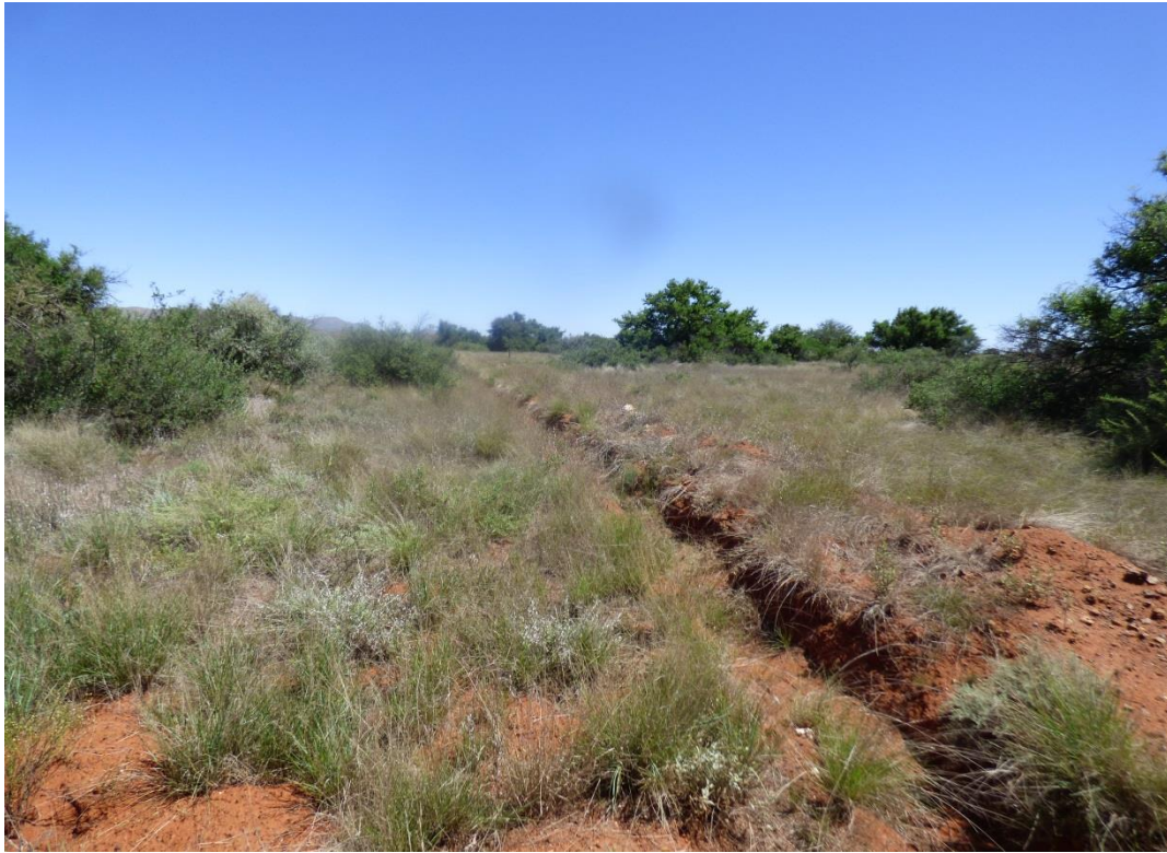
Figure 18: Irrigation pipe trench investigated for sub-surface deposits on the western footprint boundary (courtesy Ubique).
