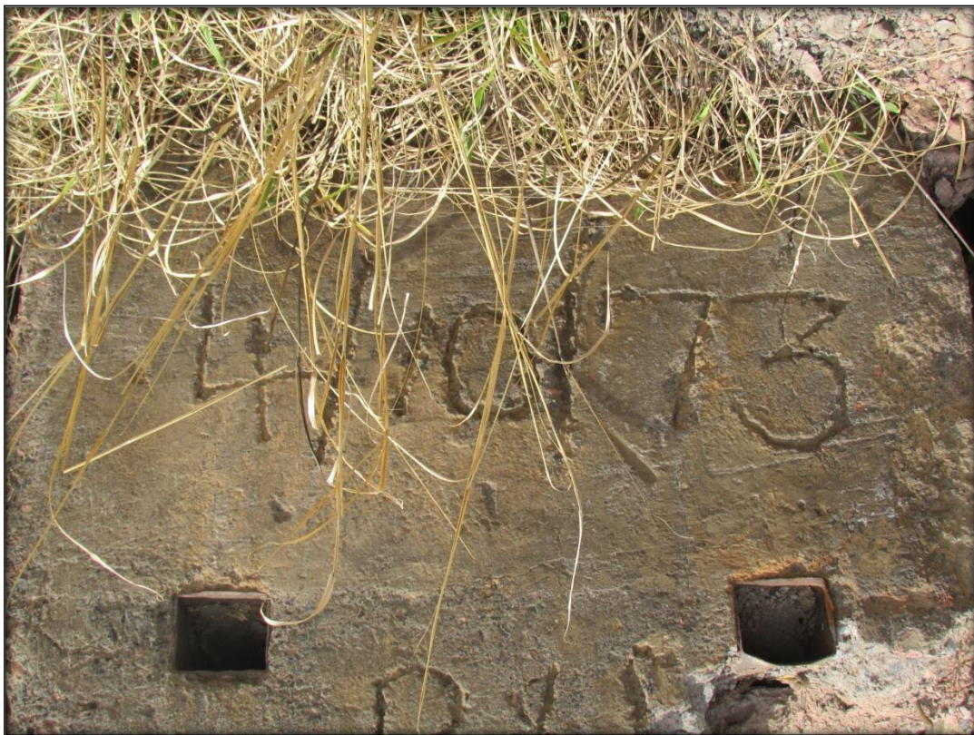
Figure 9: Picture of a cement block with a date indicating that the structures located here date to around the early 1970's.
