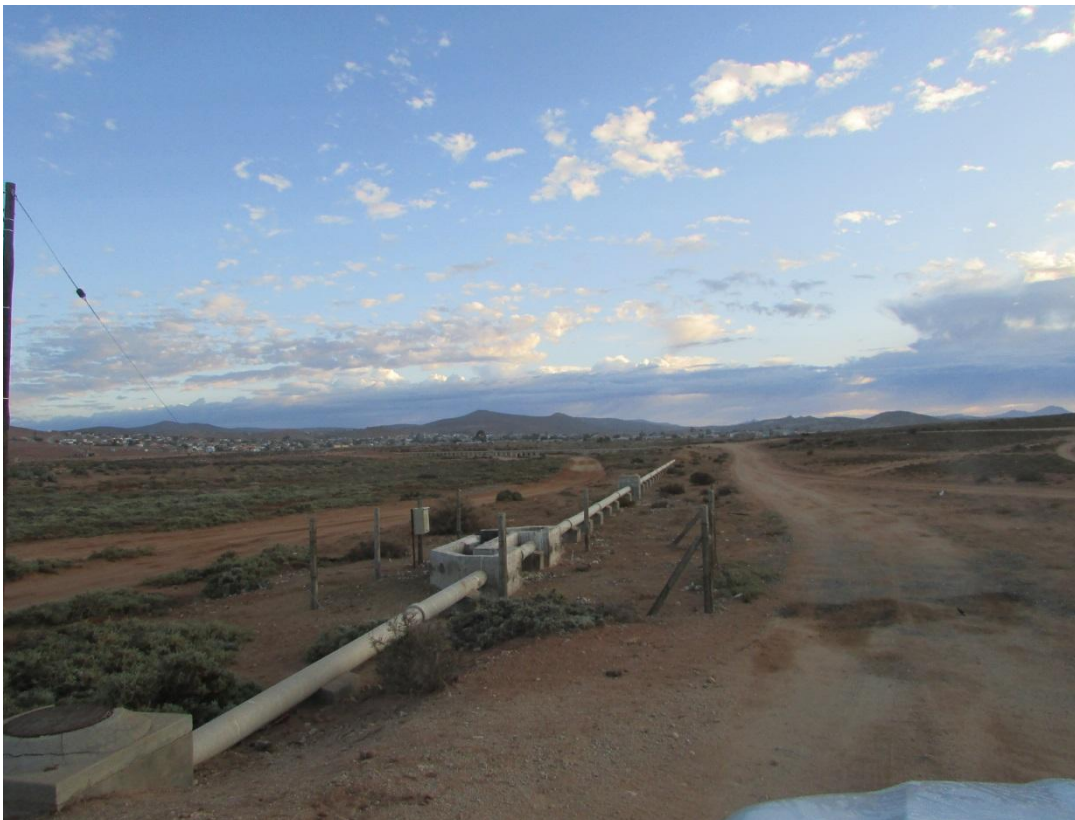
Figure 7: A view of the water pipeline that runs through a section of the area.
