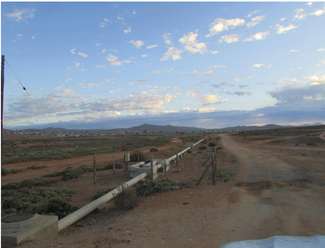
Figure 7: A view of the water pipeline that runs through a section of the area.
