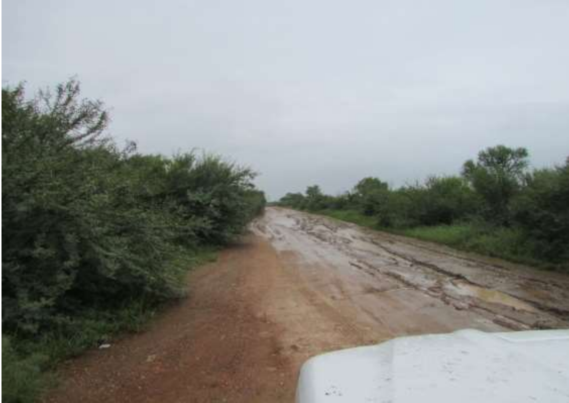
Figure 13: Sections of the route was impassable.
