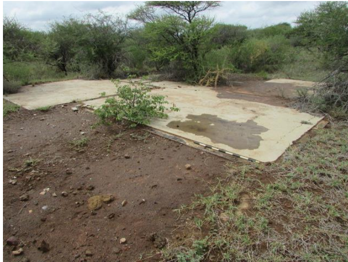
Figure 21: A view of the foundations of one of the structures on Site 2.
