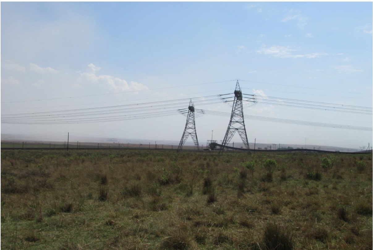
Figure 13: Impacts on the area include Eskom Powerlines.
