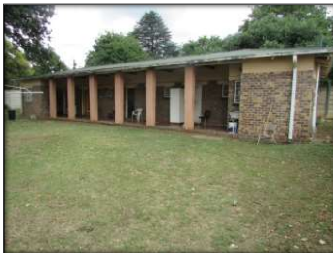
Fig.12: These recent structures will also be removed.
