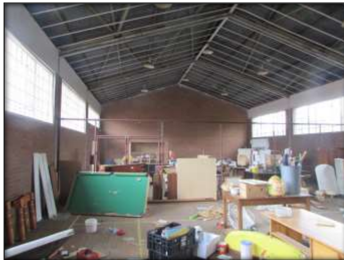
Fig.17: View of shed/storage area (old Gynasium) The structure will be retained and renovated.
