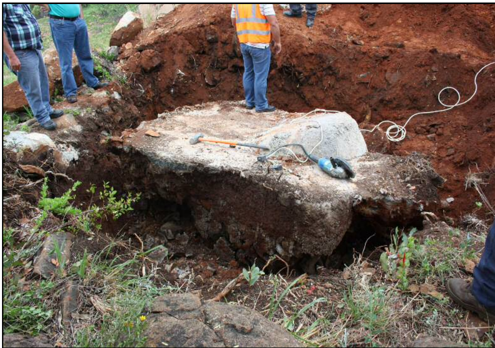
Figure 10: Removal of 1m concrete slab inside the stone wall enclosure unit 1, here Grinding and TLB machines were used to cut and remove the concrete slab in order to investigate allegation by Pakaneng Choma Community (PCC) that during the excavation of the area Roshcon came across human remains and hid them underneath the concrete. No human or animal bones were retrieved.
