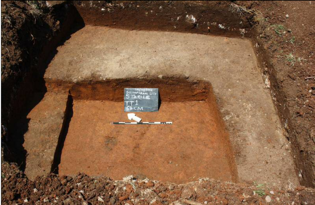
Figure 8: View of the sterile soil encountered after the removal of concrete rubble
