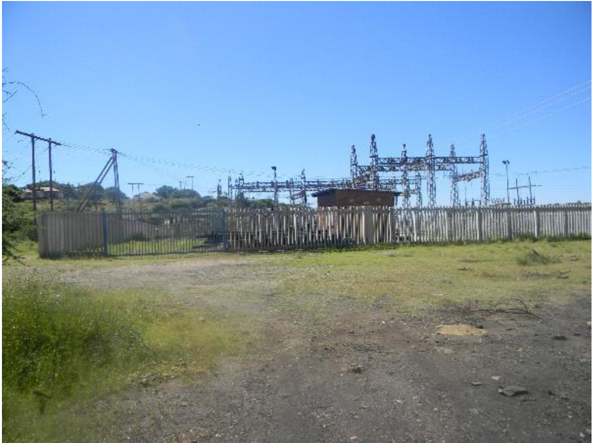
View of Norlin substation where the proposed powerline will T.OFF
