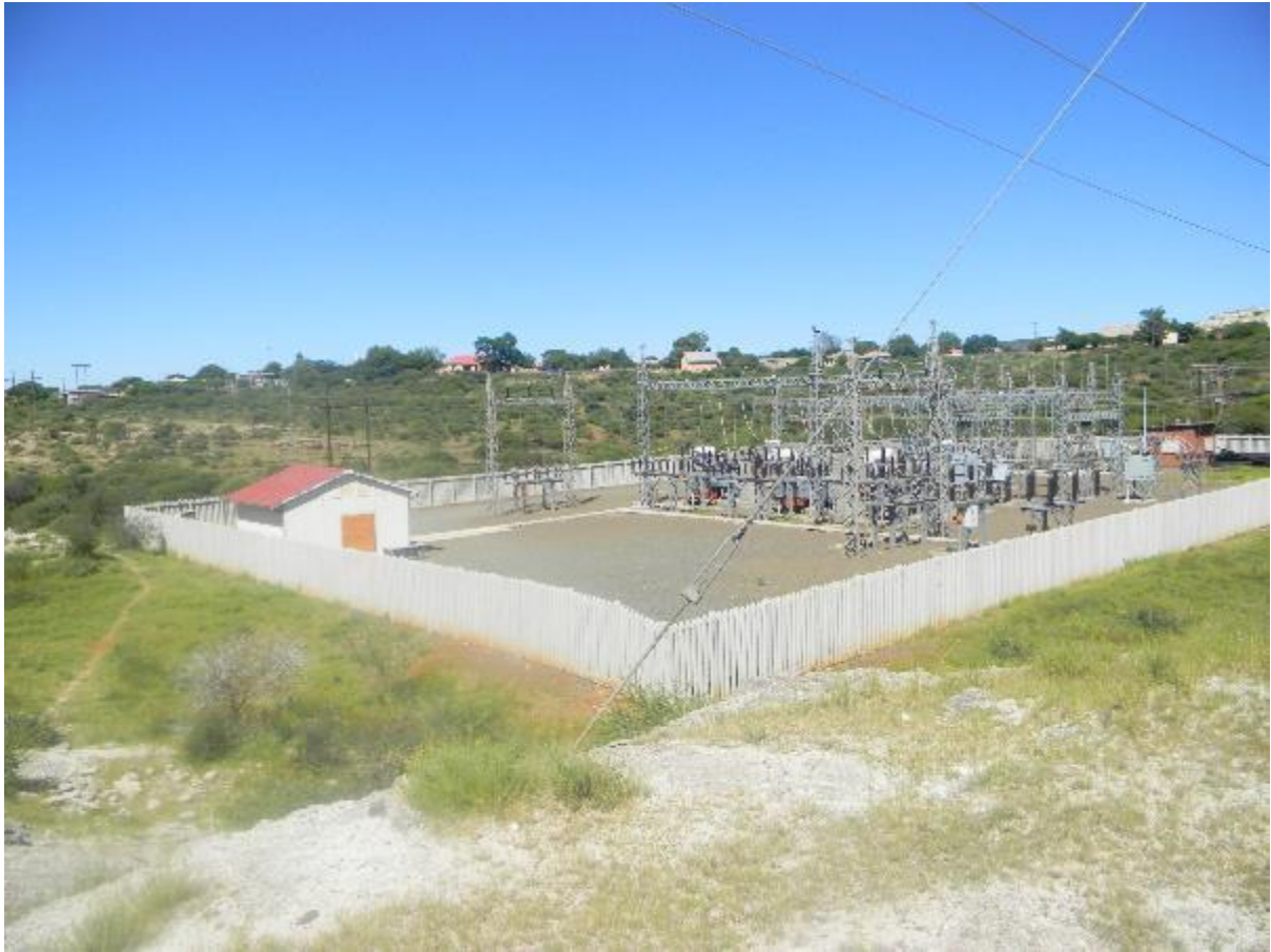
View of Norlin substation where the proposed lines will T-off from
