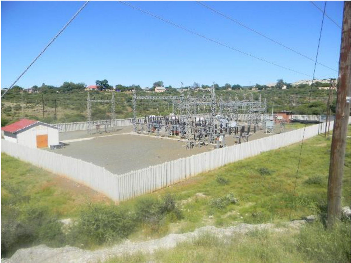
Norlin Substation where the proposed powerlines will T-off
