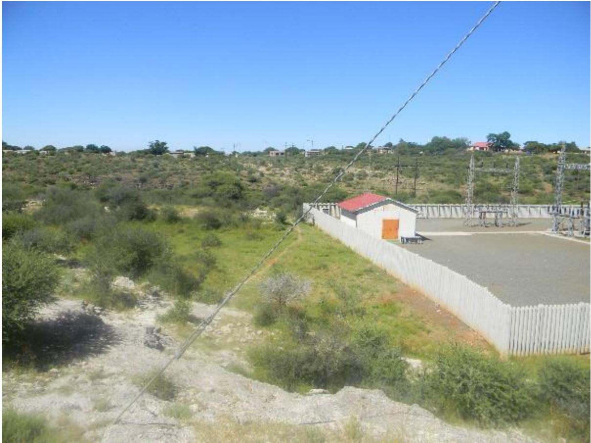
A clearer view of proposed powerline. Note that the entire project area is heavily disturbed from previous mining activities, mine residential area and encroaching
