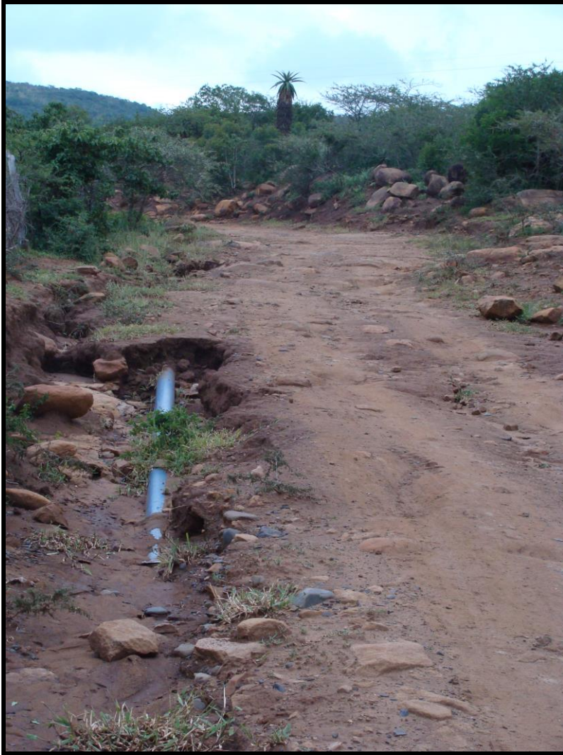
Figure 58: A pipe eroding out of the ground along the route of the pipeline as it leads up to one of the sites of the proposed reservoirs. This indicates that the underlying geology has already been disturbed during the construction of these features (GPS co-ordinates S 27° 44' 20.1" E 31° 43' 54.4")
