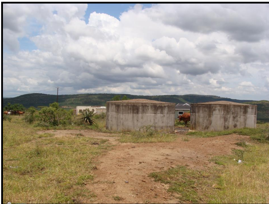
Figure 31: Small dams which will be improved and upgraded as part of the proposed project (GPS co-ordinates S 27° 53' 22.1" E 31° 51' 39.3")
