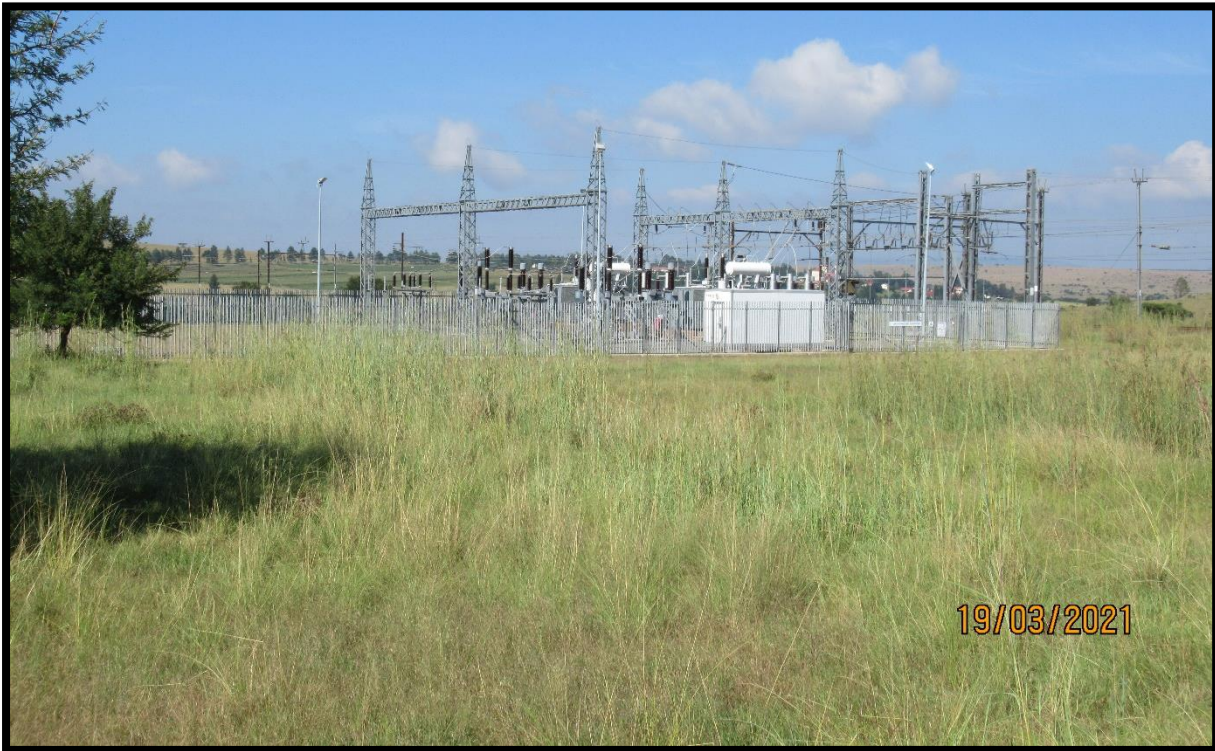
Figure 14: View of substation for the Vryheid 2 x 88 kV Turn-in Power Line with the Nzalo - Vryheid East 538 m and the Bloedrivier – Vryheid East 1175 m.
