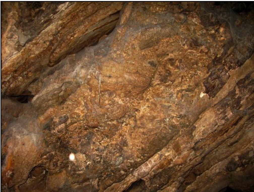
Figure 17. Side wall of upper chamber in NE showing thick (c. 1m) horizon of well-cemented early dolomite breccia that is apparently sandwiched between thin-bedded, steeply-dipping dolomite beds.
