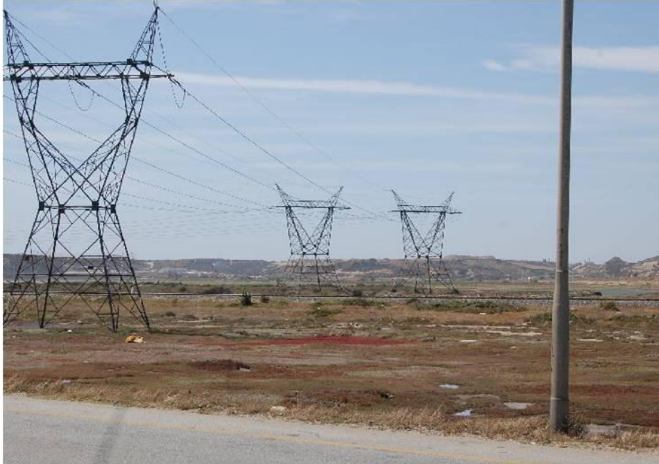
Plate 5-1: View of large power line pylons from photo site CVP009. In the background are several quarries against the hills.
