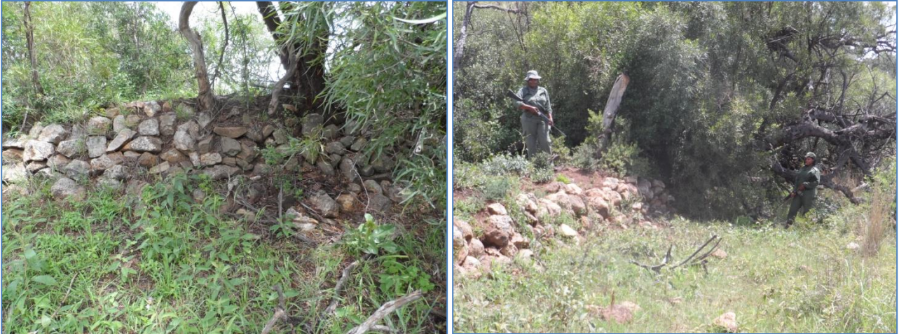
Figure 5- Stone cladded side of the dam. (Note the two Nature Reserve rangers - testimony to site visit and as scale for the height of the dam).
