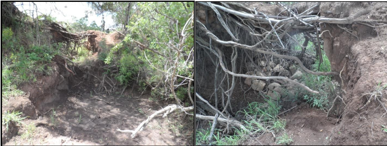
Figure 7- Soil embankment side of the dam - note the erosion which has been caused by water being channelled through the opening
