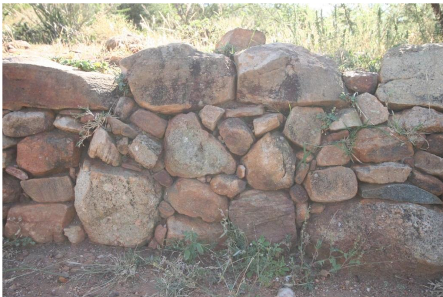
Figure 10: Retaining wall at Site S.34_05 showing level of skill and technique typical of walling in household areas higher up the slope and presumably older.
