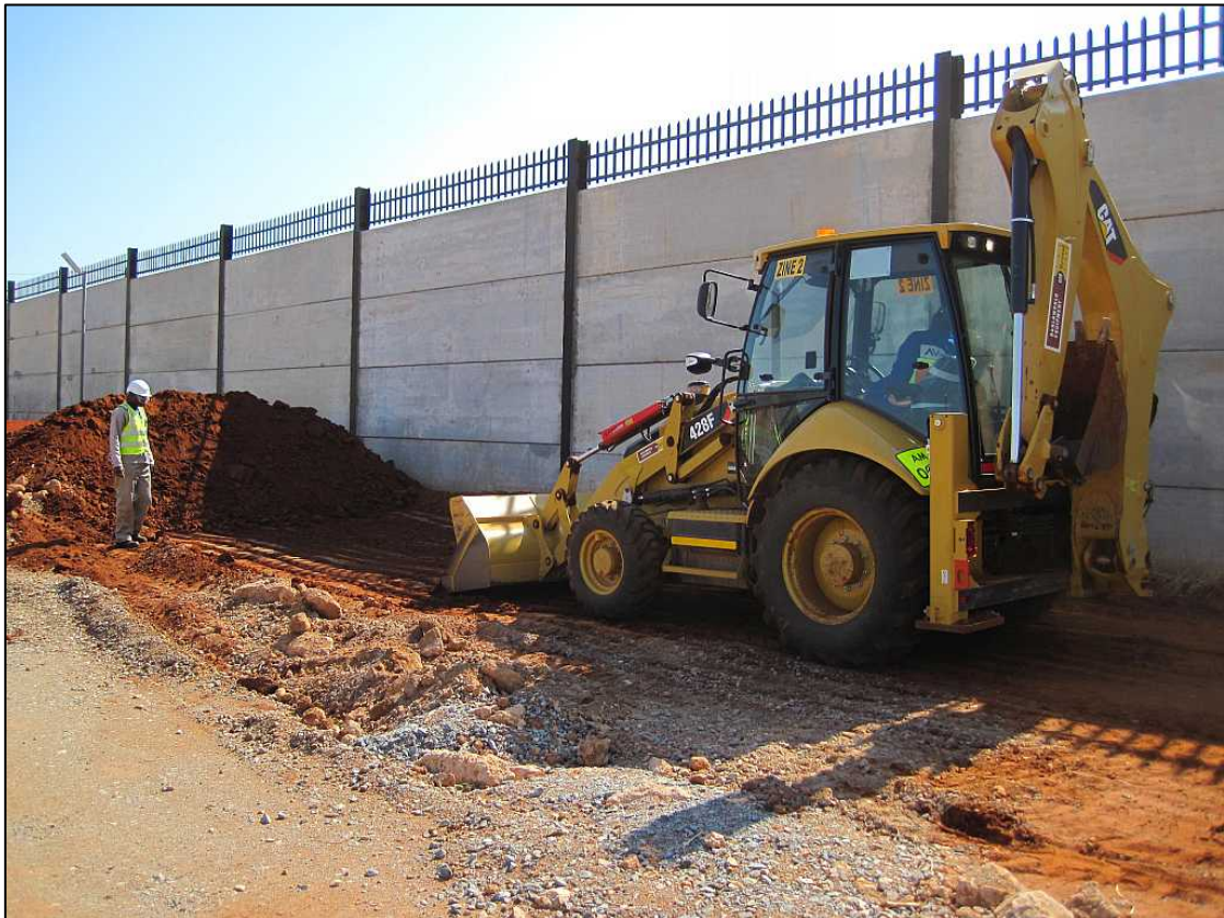
Figure 5: PGS staff supervising the TLB during the removal of the over burden and top soil.
