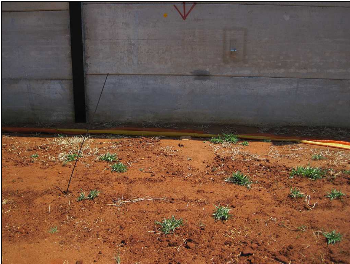
Figure 7: IVN_PGS_22_04 with the barricade partially removed on arrival before excavation work began
