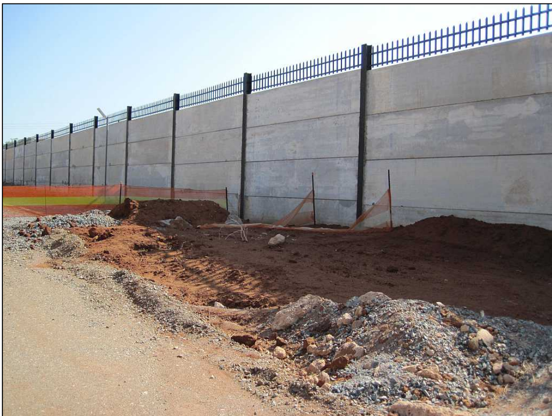
Figure 4: IVN_PGS_22_03 with the barricade partially removed on arrival before excavation work began
