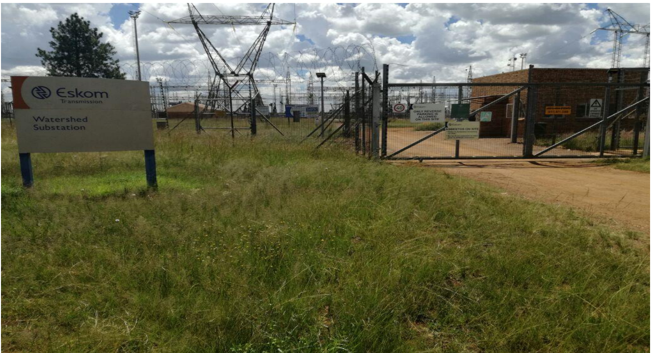
Plate 2: Photo 2: View of Watershed substation where the proposed powerline will turn to south westerly direction (Photograph © by Author 2018).
