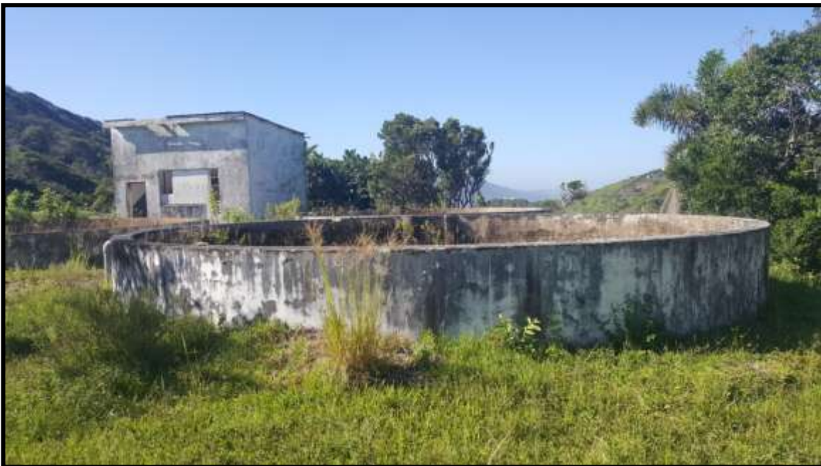
FIG. 12: WATER TREATMENT WORKS AT SITE 2
