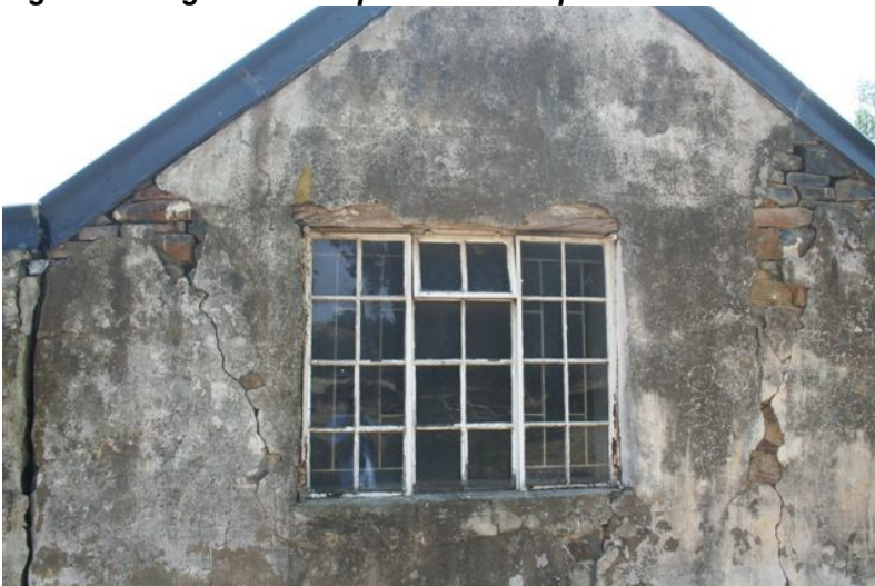
Fig 4: Showing suspected early part of house and inappropriate addition of steel windows
