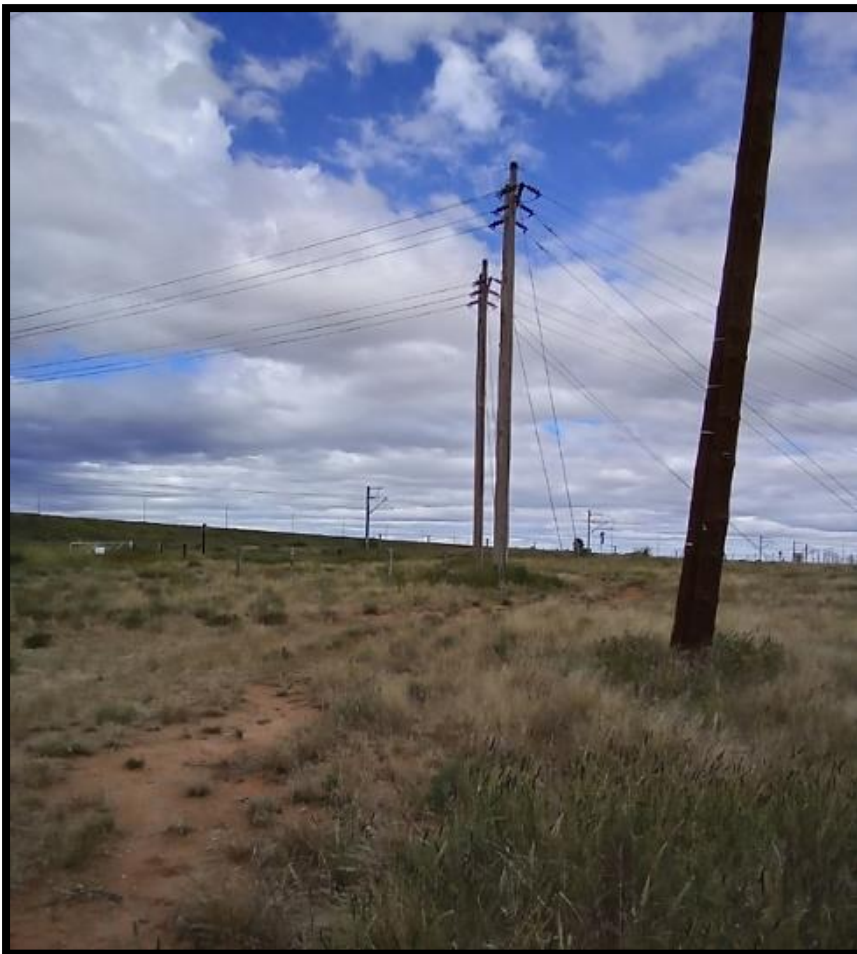
Figure 10: Existing Power lines in the south-west of the proposed Grid development corridor.
