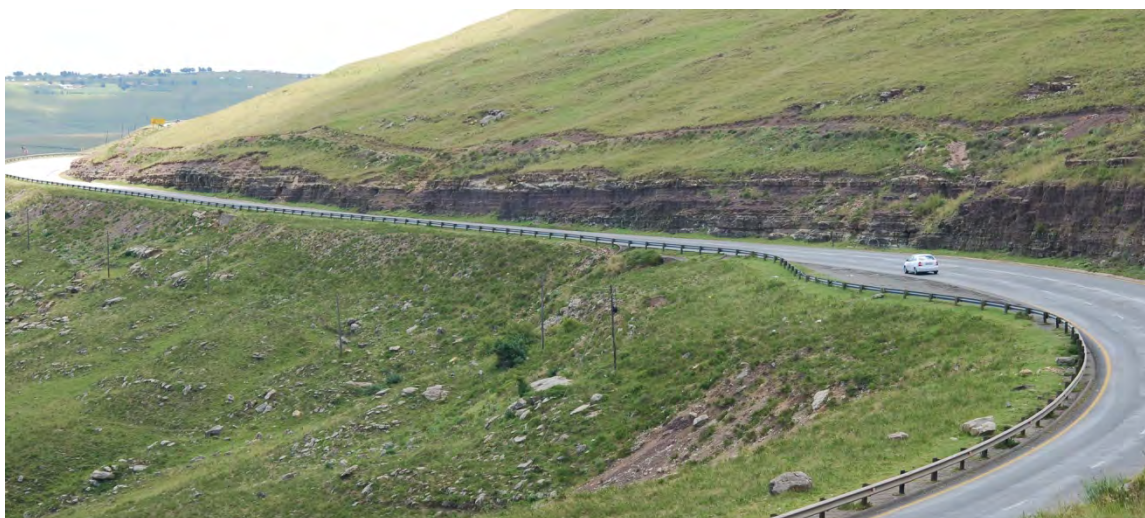
Figure 12: Katberg Formation exposed in cuttings and backdrains to the east of the Mbashe.
