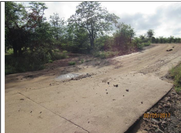
One of the many low level water river crossings over smaller drainage lines.
