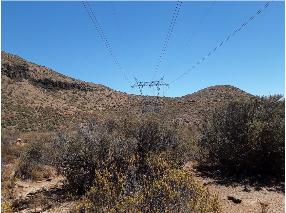
Figure 14: Existing powerline 31 ° 21' 56" S 24° 47' 57" E
