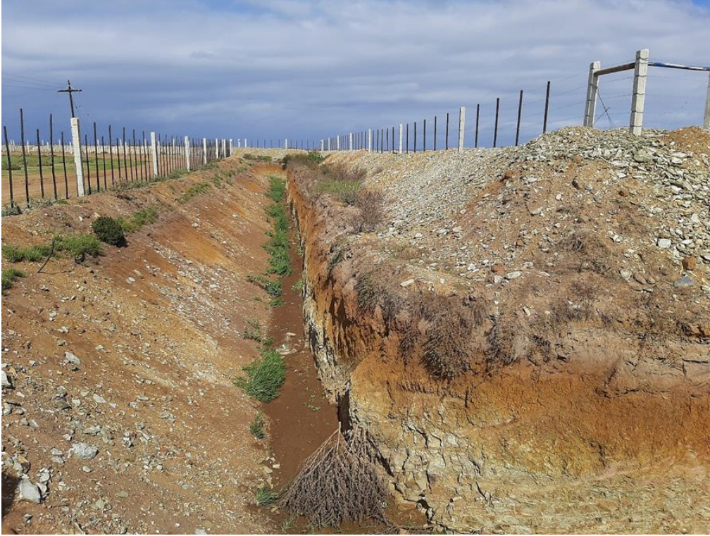
Figure 6: Soil cover and friable rock exposed in ditch next to road at 34°03'09.75"S 24°53'18.07"E
