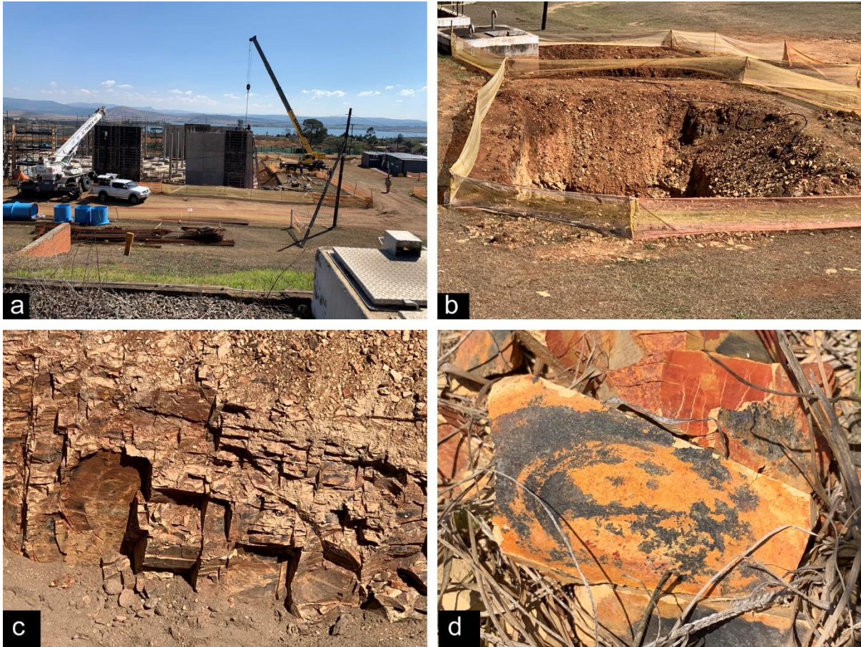
Figure 4: Photographs of the R4 reservoir area at Howick West. A – general view of construction site. B – excavation revealing the shales below the surface soils. C – fracturing and weathering of the weathered Volksrust Formation shales. D – close-up of the shales showing extreme weathering and oxidation with manganese (black) and iron (red) deposits on the fracture planes.
