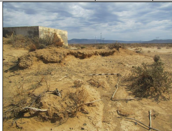
Figure 97: View of the exposed riverbank as a result of erosion.
