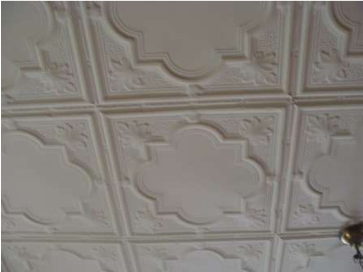
Figure 14: An example of the pressed metal ceilings found in the house. Many of the rooms has this, with each room having a different pattern.
