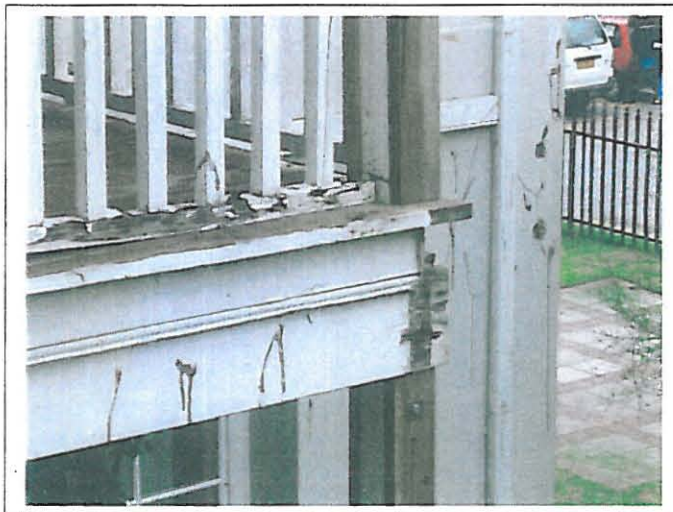
Deteriorated state of timber balustrades east facing (back) balcony.
