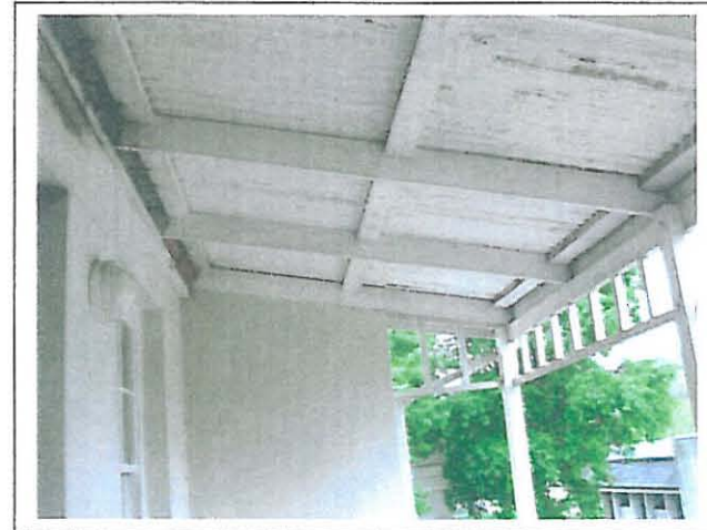
Deteriorated state of east facing (back) balcony branding board. Zinc balcony roof needs painting.
