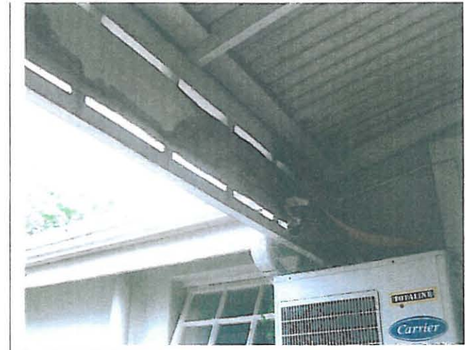
Deteriorated state of fascia board east facing (back) balcony.
