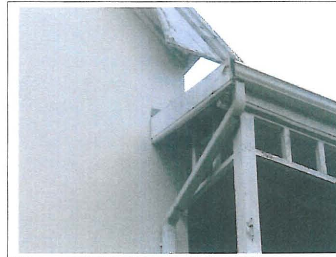
Deteriorated state of drainage down pipes and timber feature east facing (back) balcony.
