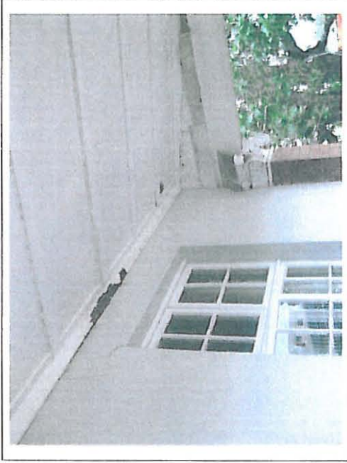
Deteriorated state of brading boards west facing (front) balcony and surface cracks in wall.
