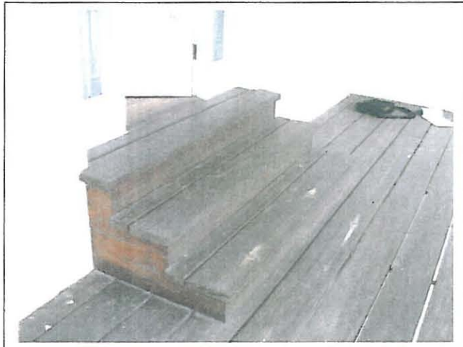
Deteriorated state of timber steps east facing (back) balcony.
