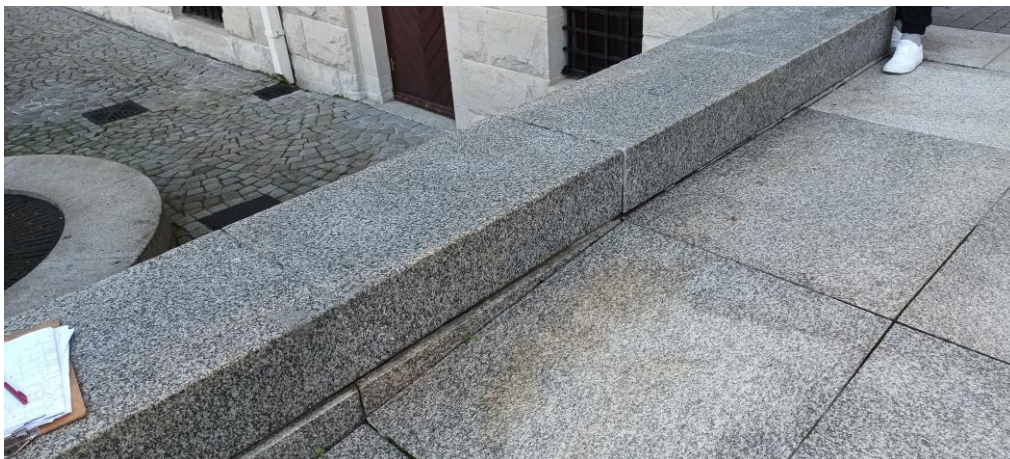
Fig 11 : Looking down from the existing ramp onto the area where the new ramp is proposed
