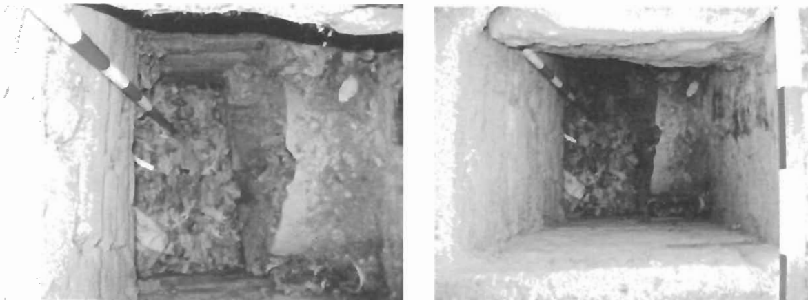
Figure 9: A close-up of the inspection chamber shows the base of the channel (clogged with leaves). The lower edge of the drain pipe sits on a ledge of bricks 1.12m below the surface level. Owing to the congestion of leaves it was not possible to measure the depth of the base of the channel. The inspection chamber was too narrow to allow for the removing the leaves.
