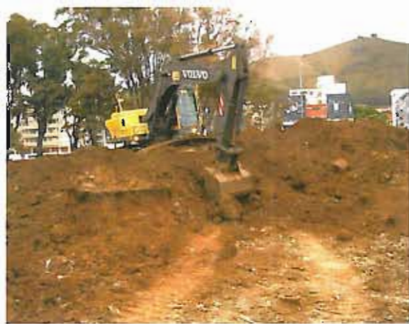
Photograph 8: Granger Bay Blvd. Excavation behind McDonald's restaurant, exposing service cables; reddish-brown soil above degraded Malmesbury shale.
