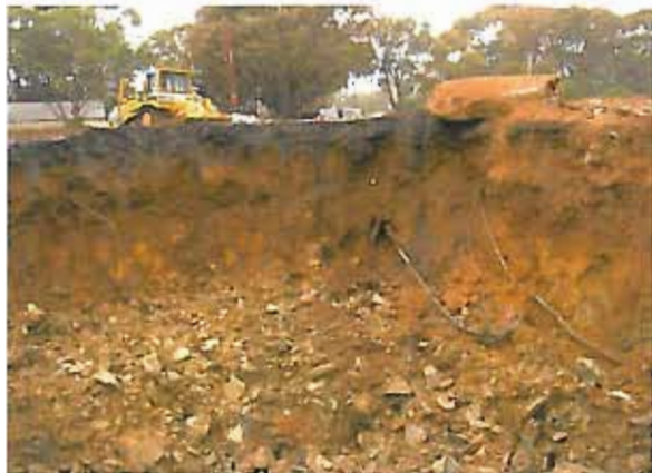
Photograph 9: Granger Bay Blvd. Excavation showing 'islands' of unexcavated material and original land surface.
