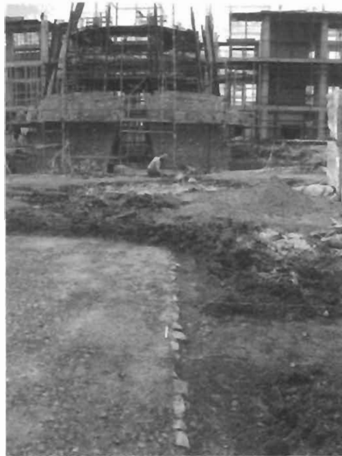
Figure 10. Photograph showing the line of edging stones marking the eastern edge of the road in Area II in the foreground.
