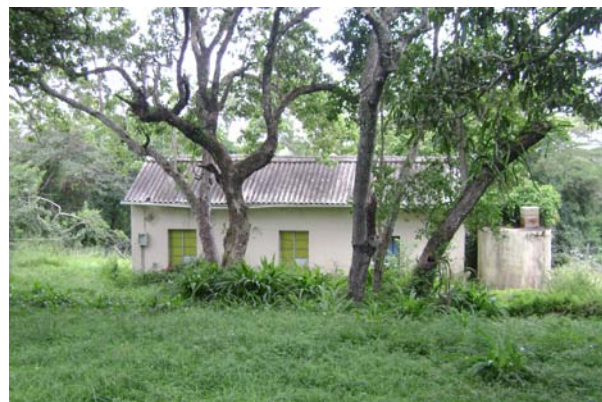
Fig 46: derelict building no 5
