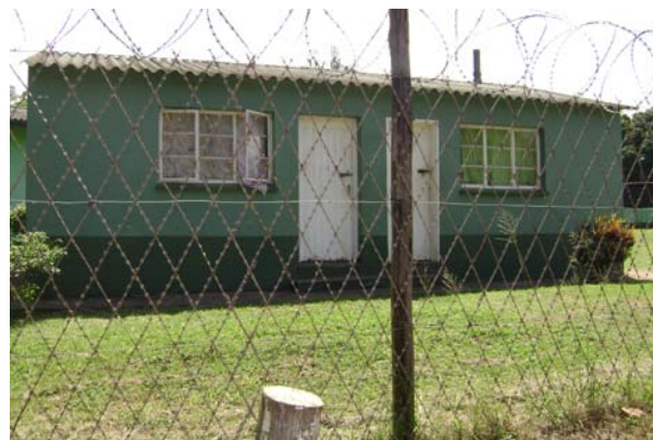
Fig 53: view of unit
