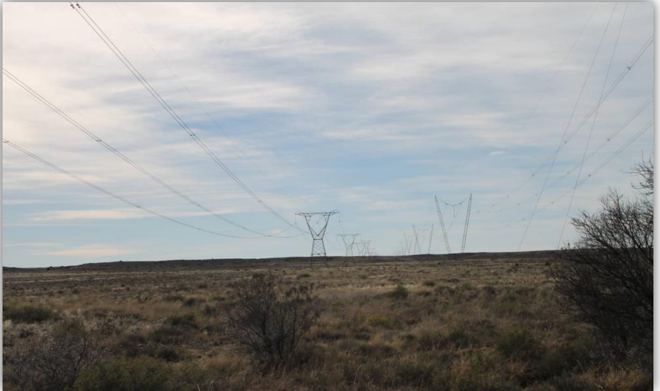
Figure 3 An example to two kinds of 400 kV lines and towers. Left: conventional self-supporting towers. Right: guyed "V" towers or compact cross-rope towers. Guyed "V" towers have a very small ground surface footprint and are more easily absorbed against a skyline.
