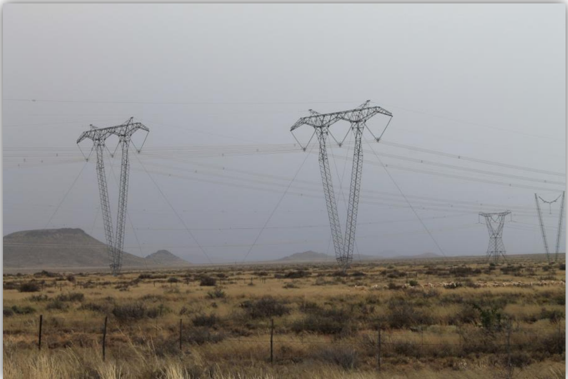
Figure 4 A set of new 765 kV transmission lines north of De Aar (Perseus-Hydra). They are substantially taller than the 400 kV lines in the background.
