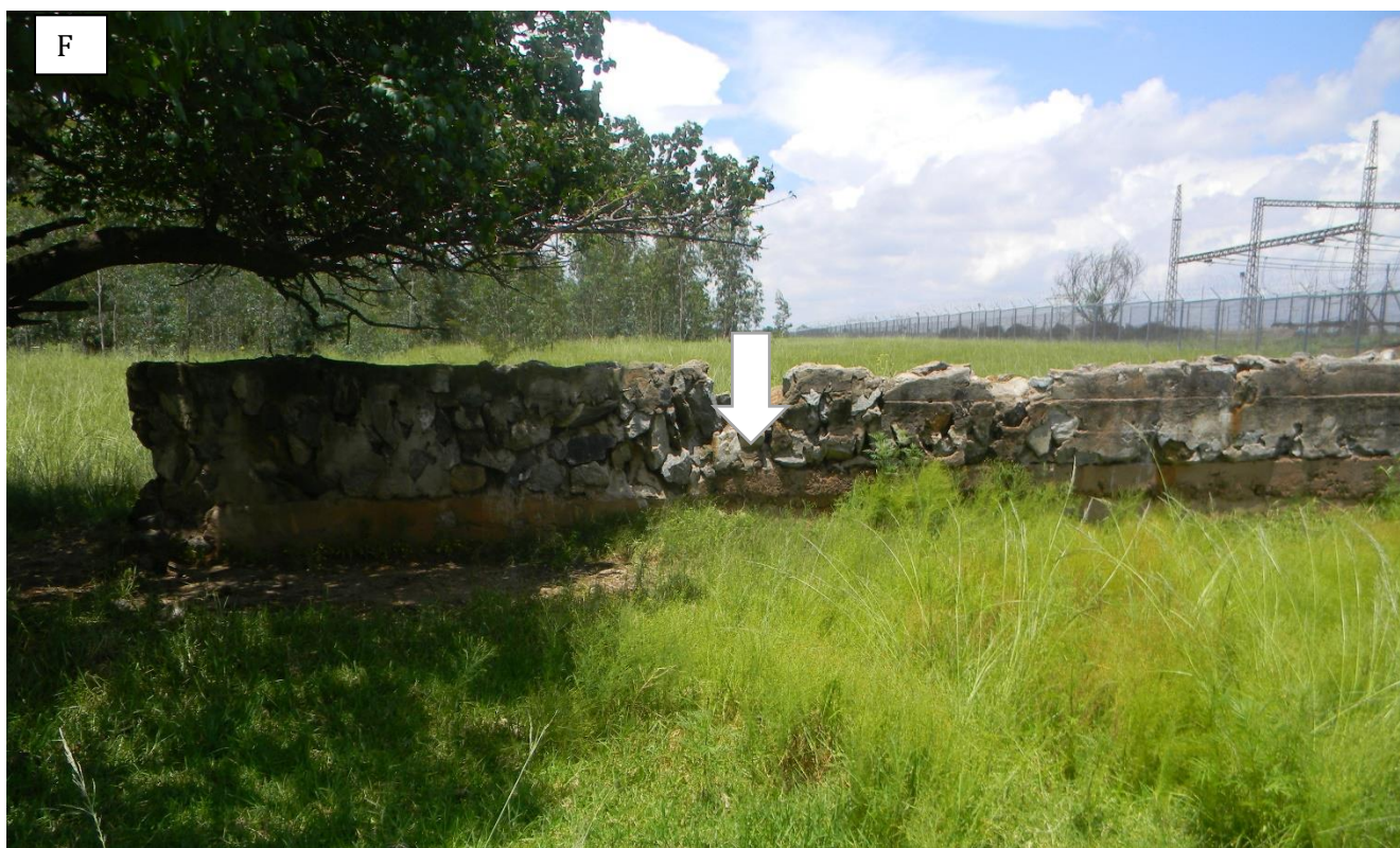
Plate 6: Photo F showing remains of perimeter wall/kraal with signs of collapsing.
