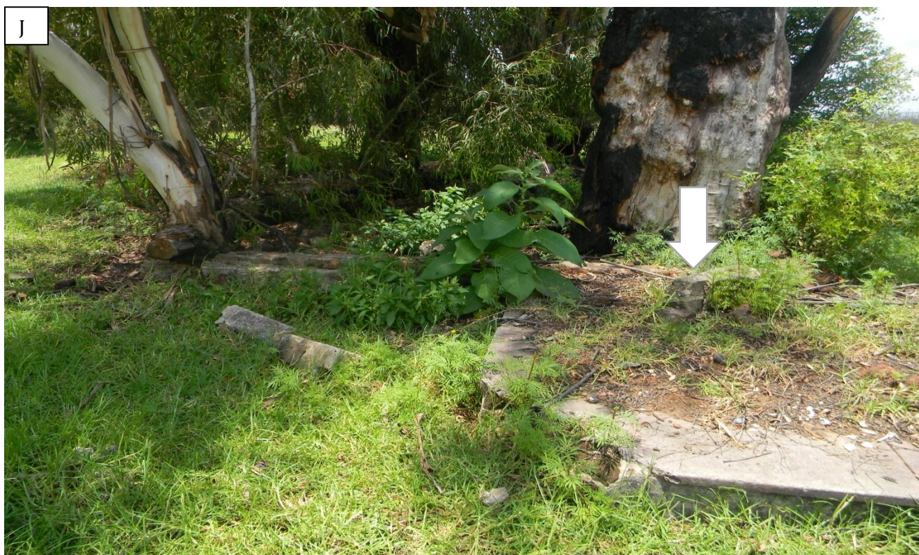
Plate 10: Photo J, showing overgrown vegetation that affected remains of house foundation and floors.
