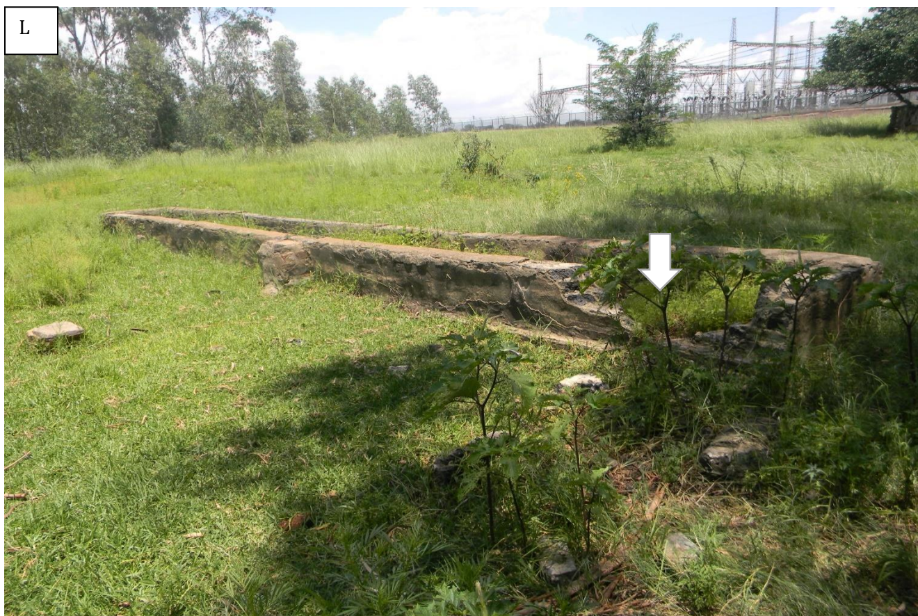
Plate 12: Photo L, showing partially vandalised wall of the livestock drinking trough.
