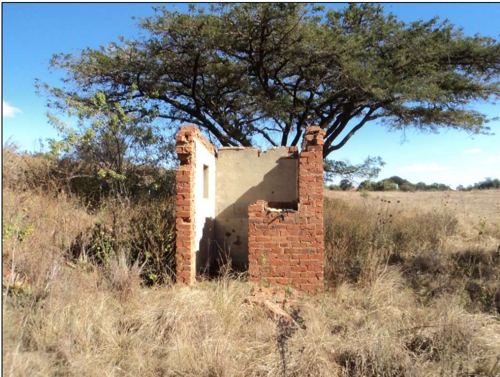
Figure 40: Dilapidated toilet building at Site K13.
