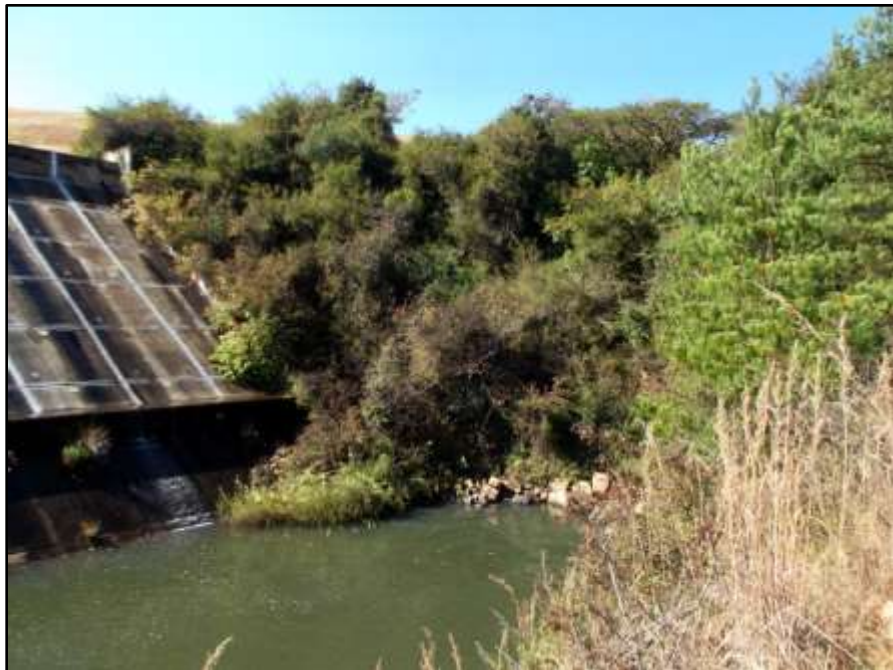
Fig. 12. Site SO 6. The southern side of the spillway. Construction site 1 proposed to the right thereof.
