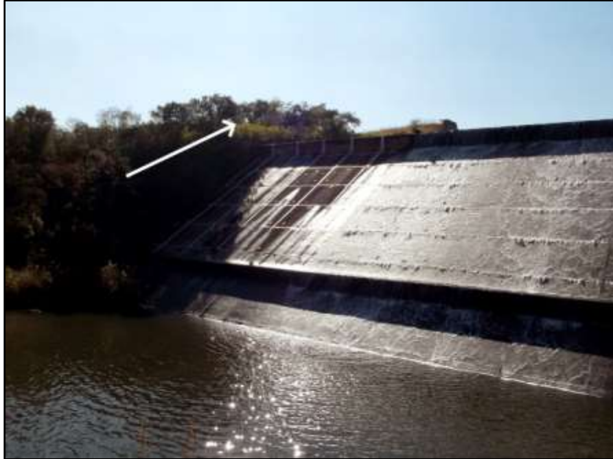
Fig. 11. Site SO 6. The current dam spillway. The arrow indicates the fuseplug embankment which will be elevated as part of the proposed remedial work. Photo taken in a north-eastern direction.
