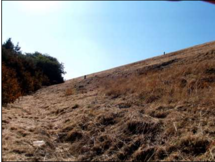
Fig. 7. Site SO 4. The western side of the dam wall/ embankment Photo taken in a northern direction.
