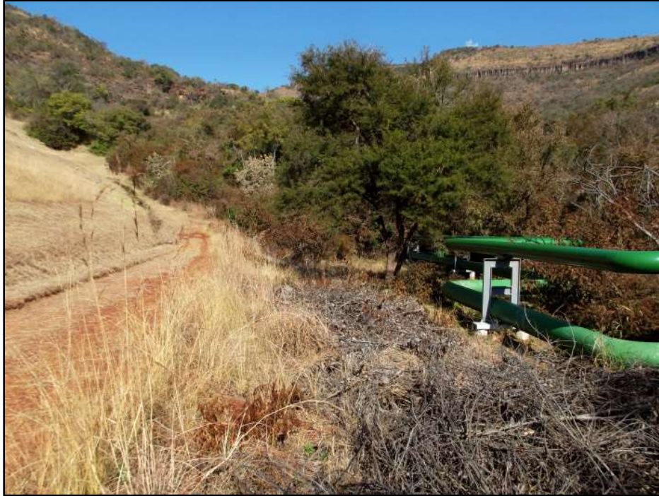
Fig. 15. Site SO 7. Photo taken south. The access road proposed to widen and stabilizing berm to be constructed. To the left is the current dam wall or embankment.
