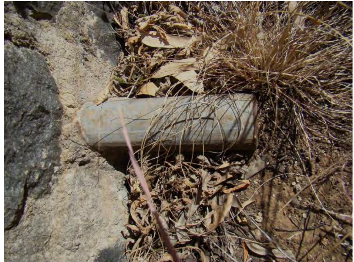
Figure 49: Metal outlet pipe
