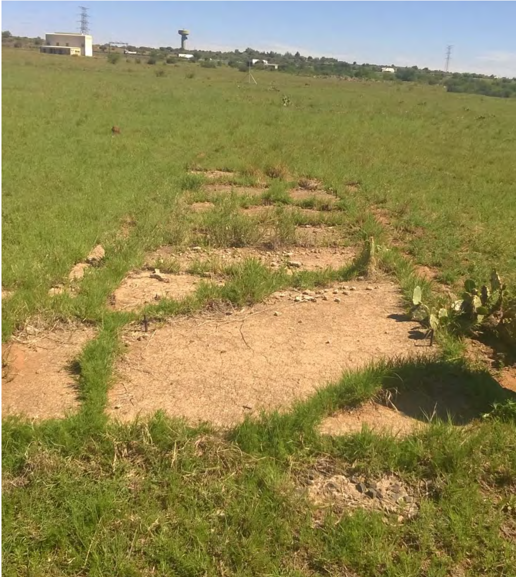
Figure 38: Severely eroded foundation
