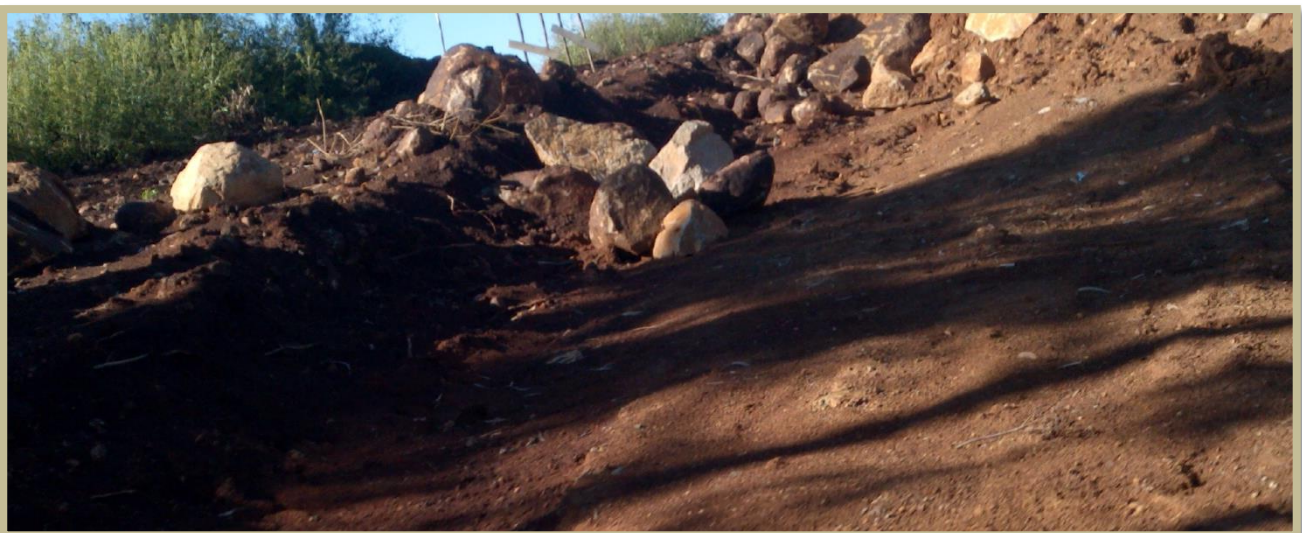
Figure 6 Deeply weathered overburden with dolerite inclusions in new cuttings for access ramps
